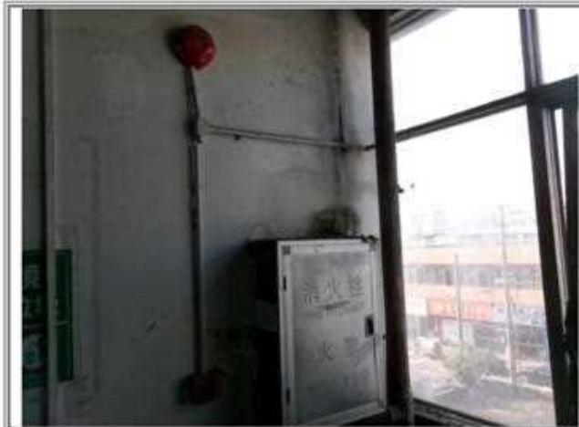
Fire hydrant and fire alarm
