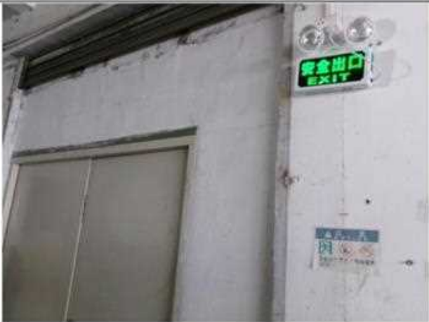
Exit sign and emergency light above emergency exit
